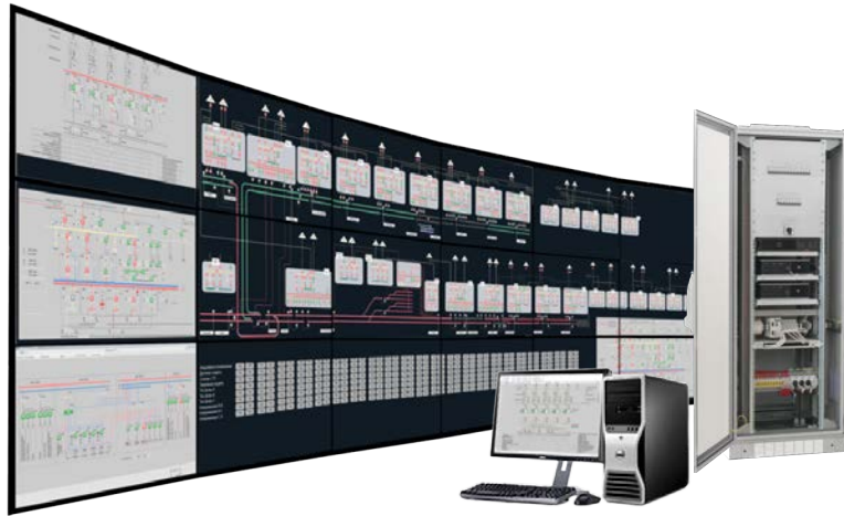
3 rd level. Operator control
