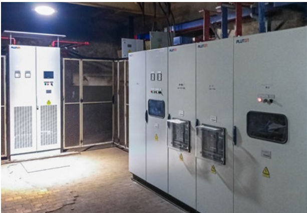
Ukraine, Zaporizhstal steel works two-unit KVPP-4.0k-230
