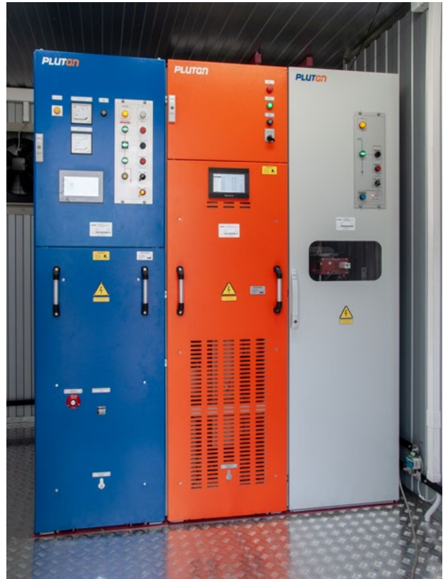
▲ Negative busbar switchgear (on the right), withdrawable rectifier (in the middle) DC switchgear (on the left)
